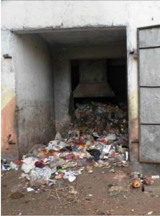
Figure 5: The garbage dump which requires a new door
